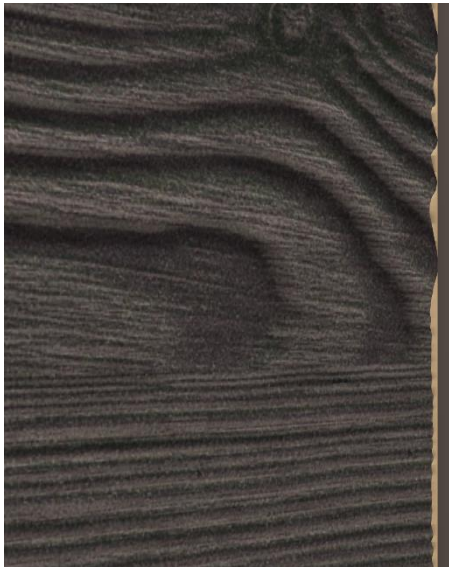
Fig. 6 – Damaged surface layer –
